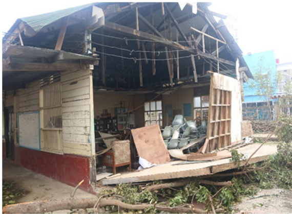
Fig. 12. Toppled one side wall of an old building in the university.
