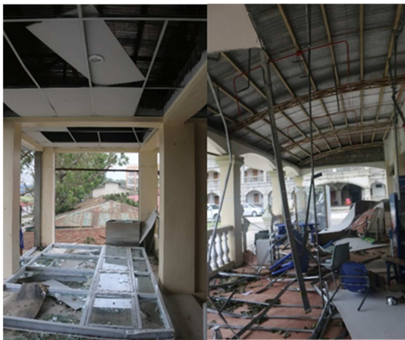
Fig. 13. Blown off glass walls (left) and outside debris of Research Development and Extension Building and left part of the Gymnasium used as canteen.
