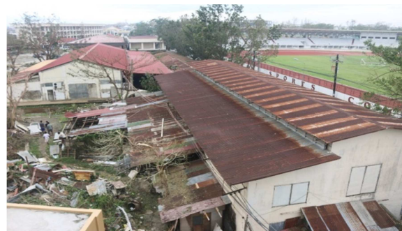
Fig. 10. Peeled-off roof and blown off debris after the disaster Typhoon Ompong.
