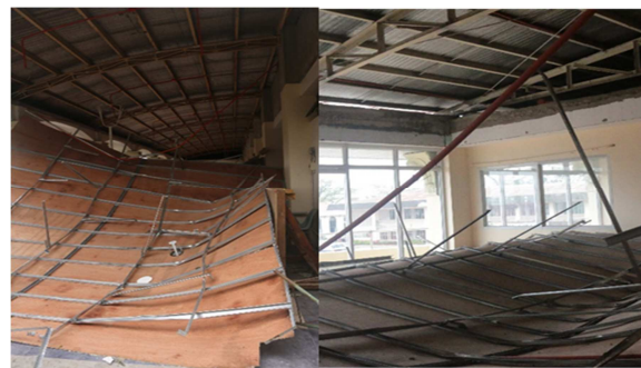
Fig. 11. Collapse ceiling revealing roof truss and roofing sheet after the typhoon.
