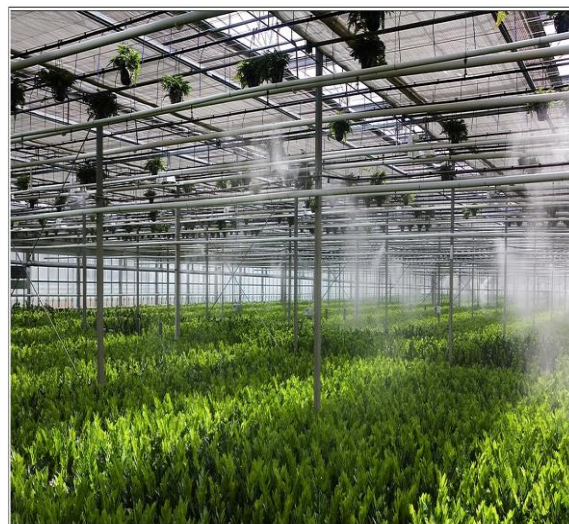
Fig. 7. Fogging system in green house.
