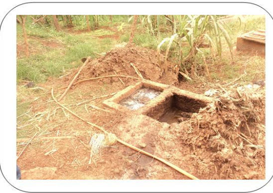
Fig. 2. Biogas plant at Viti village indicates poor management that lead to low gas production and destruction of the plant system.
