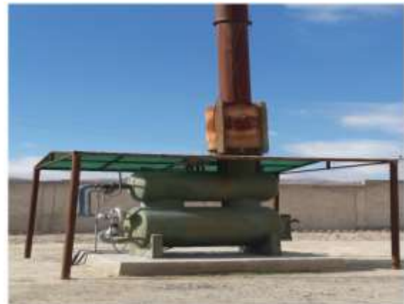
Fig. 3. Incinerator installed at Bolan Medical Complex.
